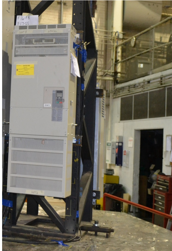
All units were filled with contents and maintained structural integrity and functionality
